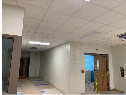
Ceiling Tile in Building 2033
