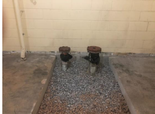
Fire Department Connection
