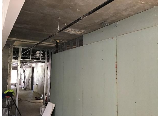
Building 2032 Sprinkler Piping
