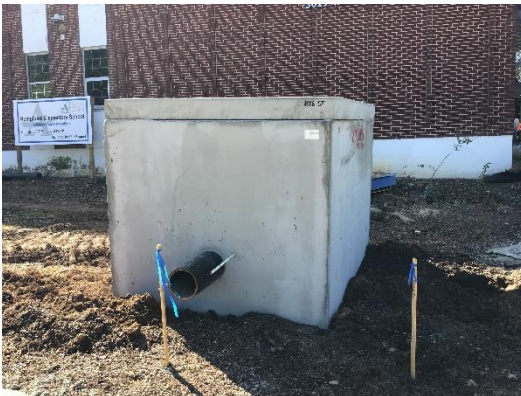
Domestic Water Meter Vault
