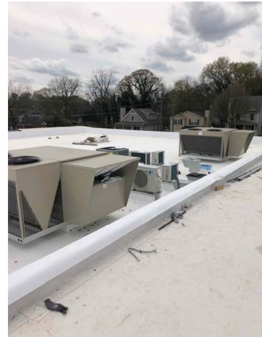
New gym HVAC equipment
