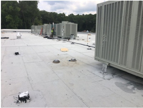
Gas piping to Tower Units at WPA
