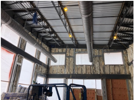
Spiral Duct at YMCA
