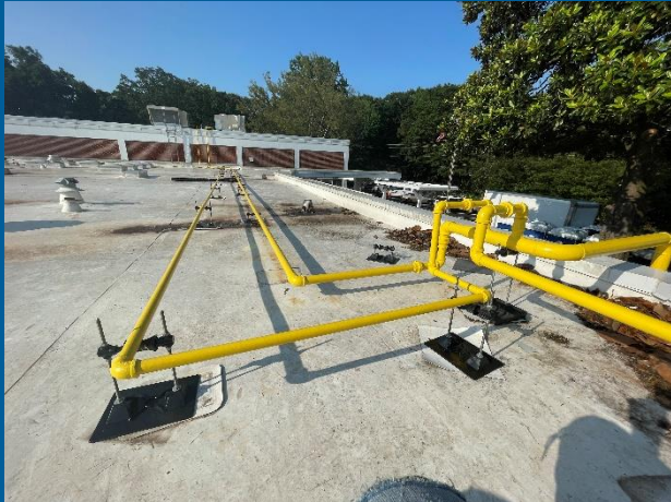
Painted Gas line
