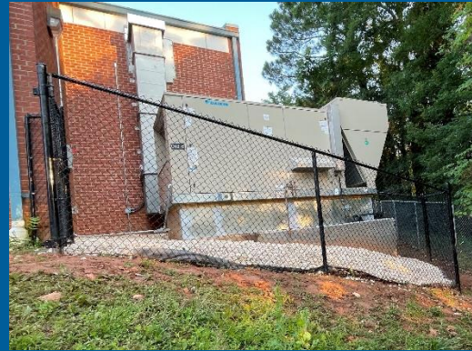
River rock gravel around ground HVAC Units
