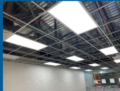
Lights Set in Gym Ceiling Grid
