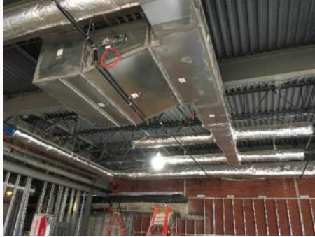
HVAC at Kitchen/Cafe Tie-In to AHU
