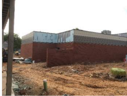
Can Wash Wall & Metal Panels
