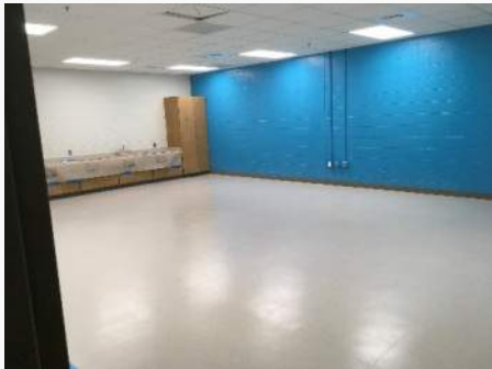
VCT Waxing & Wall Base at Reno Typical Classroom
