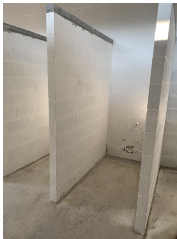
FD-1st Coat Paint
