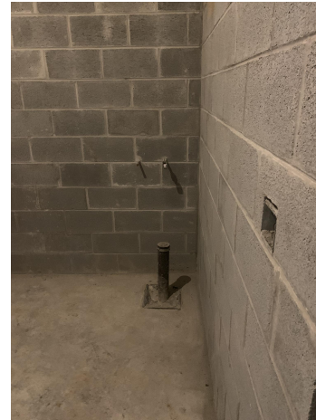
FD-Mechanical room prep
