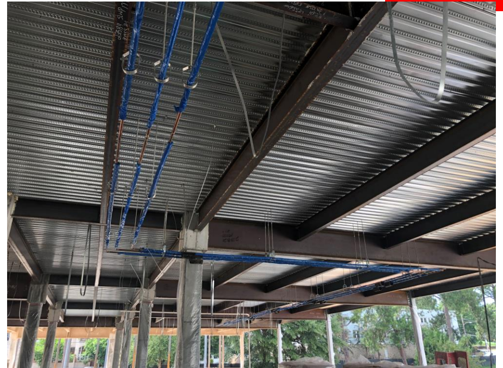
Second Floor Plumbing Overhead
